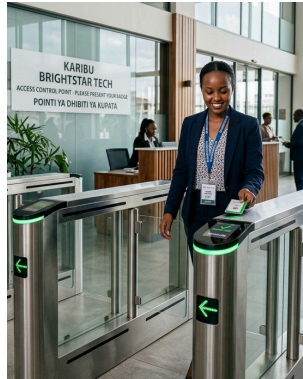
Smart door and gate access control
